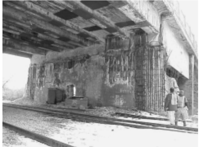
The aging Rockefeller Road Bridge, Cleveland, Ohio, is one of many decaying bridges over the rail corridor.
