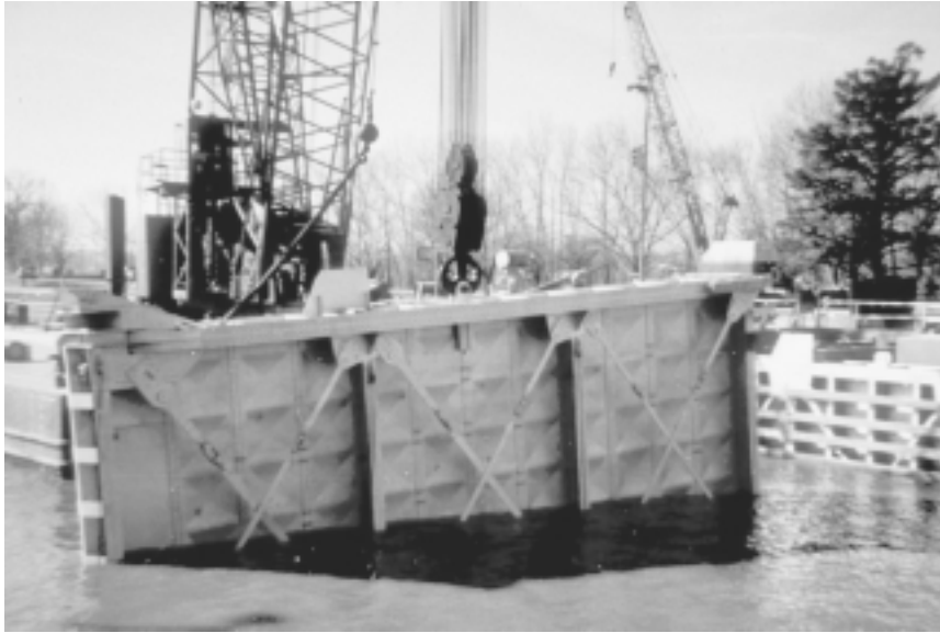
The crane “Quad Cities” here lowers into position a temporary gate, in the lower gates of the main chamber at Lock and Dam 15, on the Mississippi River, in Rock Island, Illinois, to replace a cracked structure removed for repairs off-site. This is the last temporary gate the Army Corps of Engineers has available for emergency use on the Mississippi.
