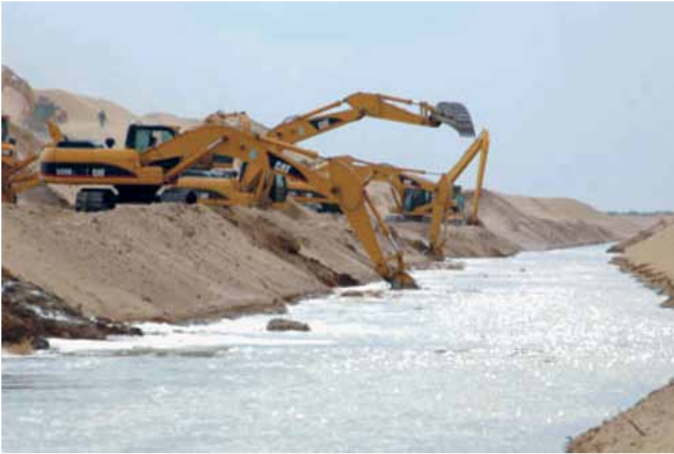
One of the canals feeding the Altyn Asyr artificial lake during construction.
