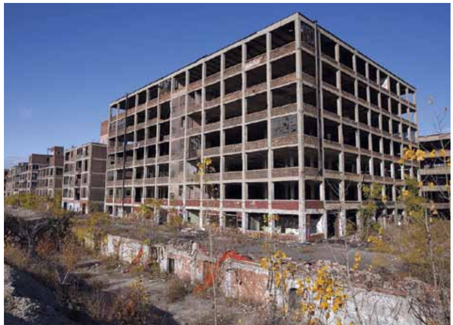
All the jobs are gone. How do we move beyond words and actually solve the problem? Here, the western part of the abandoned Packard Automotive Plant in Detroit, Michigan, in 2009.
