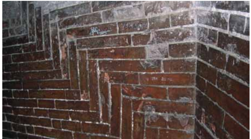
The herringbone brickwork in the space between the inner and outer domes.
