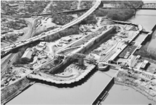
The function of LaRouche PAC will be to provide “guidelines for rebuilding the U.S. economy.” On the Ohio River there are lock systems which are “in danger of breaking up.” McAlpine Lock, on the Ohio River near Louisville, Kentucky, shown here, was closed this Summer for emergency repairs, which closed the Ohio River to barge traffic for two weeks. The outdated lock is in the process of being replaced by the U.S. Army Corps of Engineers.
