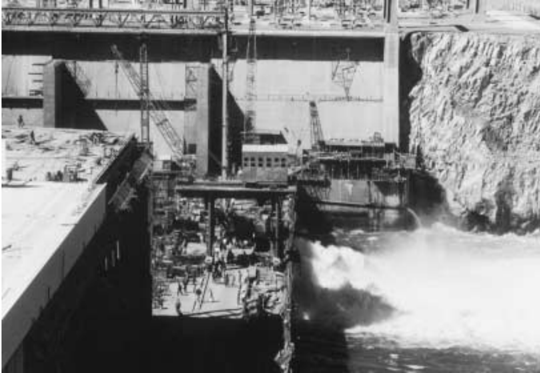
Construction of the High Aswan Dam near completion in 1968. Dr. Said convinced Nasser on a four-year (1958-62) project of mapping, geological surveying, and preservation of important sites in the area of Nubia that was to be flooded, which Dr. Said carried out, part of his decades of study of the Nile River.
