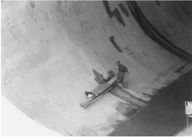
A worker is dwarfed by the size of the intake tunnels under construction for the dam.
