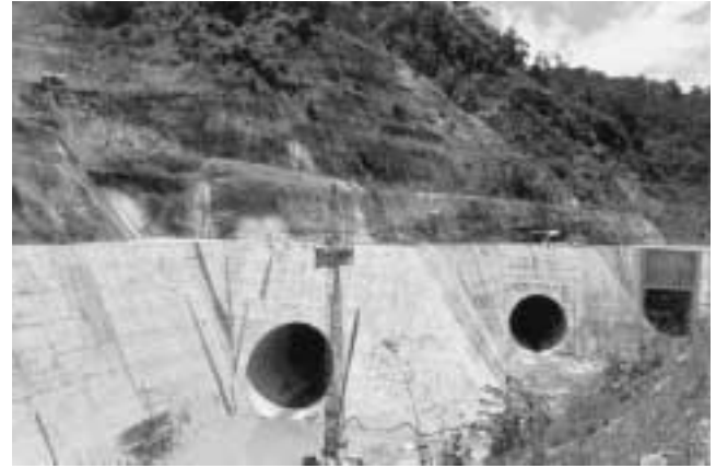
Diversion tunnels have already been drilled in preparation for the dam construction.
