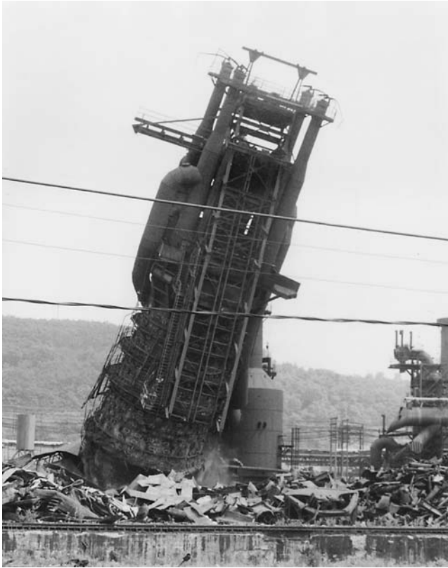
Demolition of a U.S. Steel plant in McKeesport, Pennsylvania, 1985. It is this “rust belt” phenomenon, which typifies the developments which have made the U.S. economy so vulnerable to the crisis of the region including California, today.
