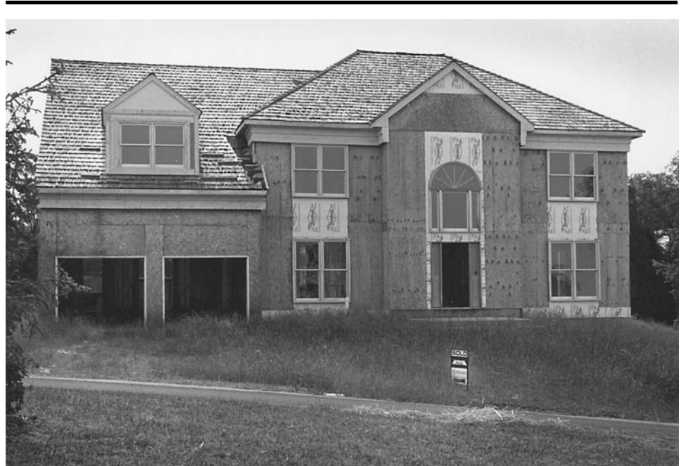
An expensive Virginia home, partly constructed, sold, foreclosed and abandoned in short order, confirms Freeman’s forecast.
