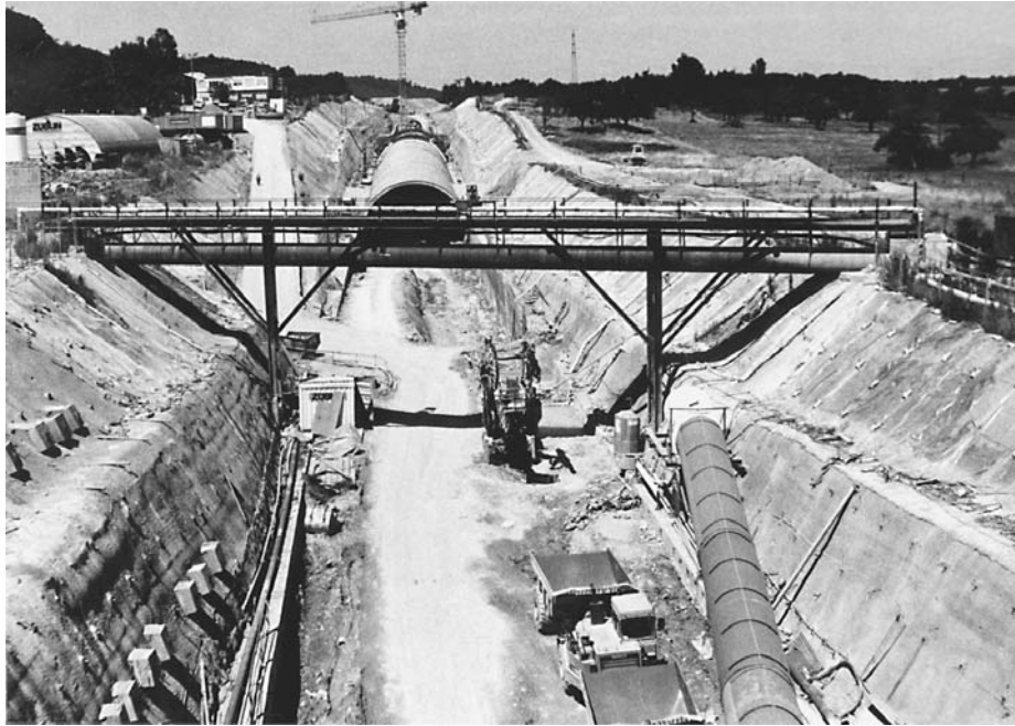
Construction of a tunnel for the ICE high-speed train in Nidenhausen, Germany.
