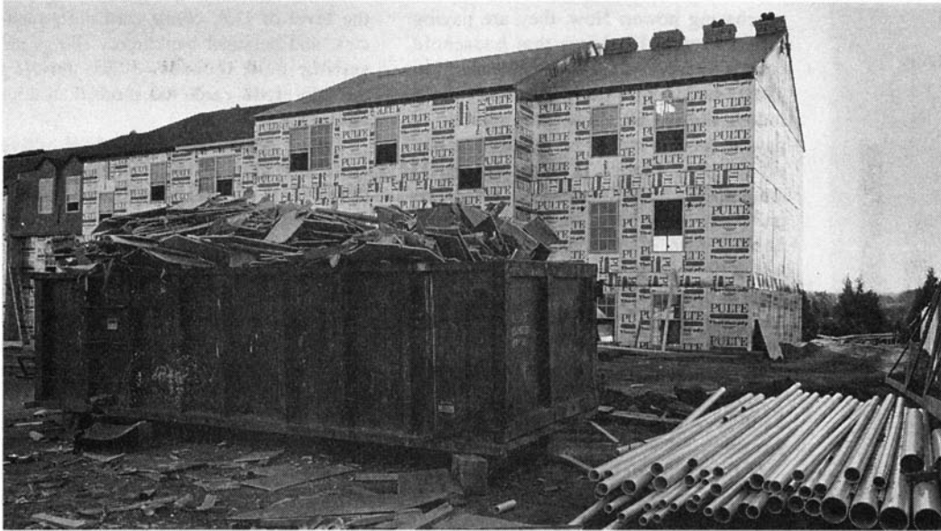
Townhouse construction in northern Virginia. Shoddy construction and cheap materials are now the order of the day throughout much of the nation's construction industry.
