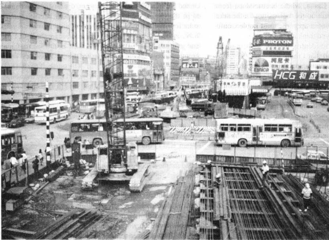
Taiwan is facing a growing political and moral crisis. This subway construction project in downtown Taipei has been reduced by half.
