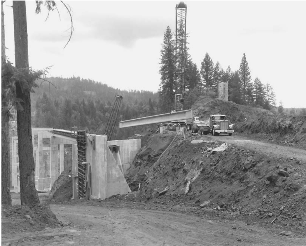
The U.S. Army Corps of Engineers works on a bridge project at Lost Creek Lake, Oregon. The Corps has a vital role to play, with cooperating non-military agencies, in conducting a large-scale development of the basic economic infrastructure of our nation, and in cooperation with other nations.
